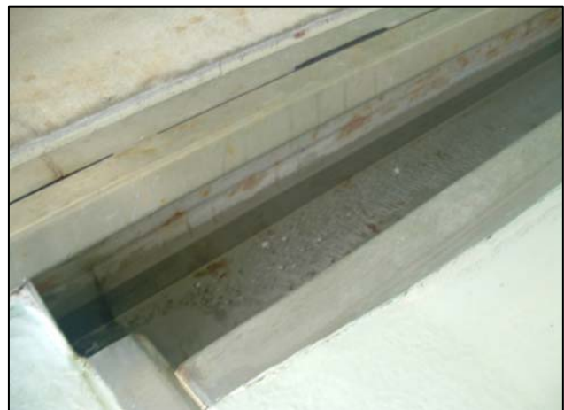
Fig 3. Sand/media in gutter trough
