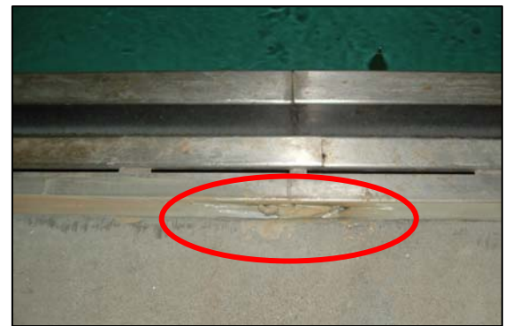
Fig 6. Gap in sealant
