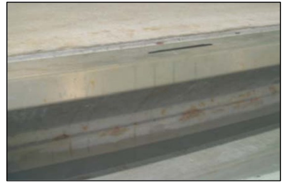
Fig 5. Corrosion in trough
